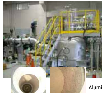
Interior view of the heater before being filled with pebbles (heat-resistant bricks can be seen on the sides and wire mesh to support the pebbles at the bottom).
